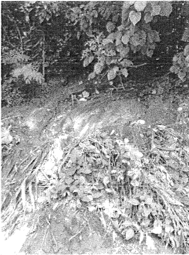
Photograph 21. Marbo Cave erosion area 2 near opening, 072821.
