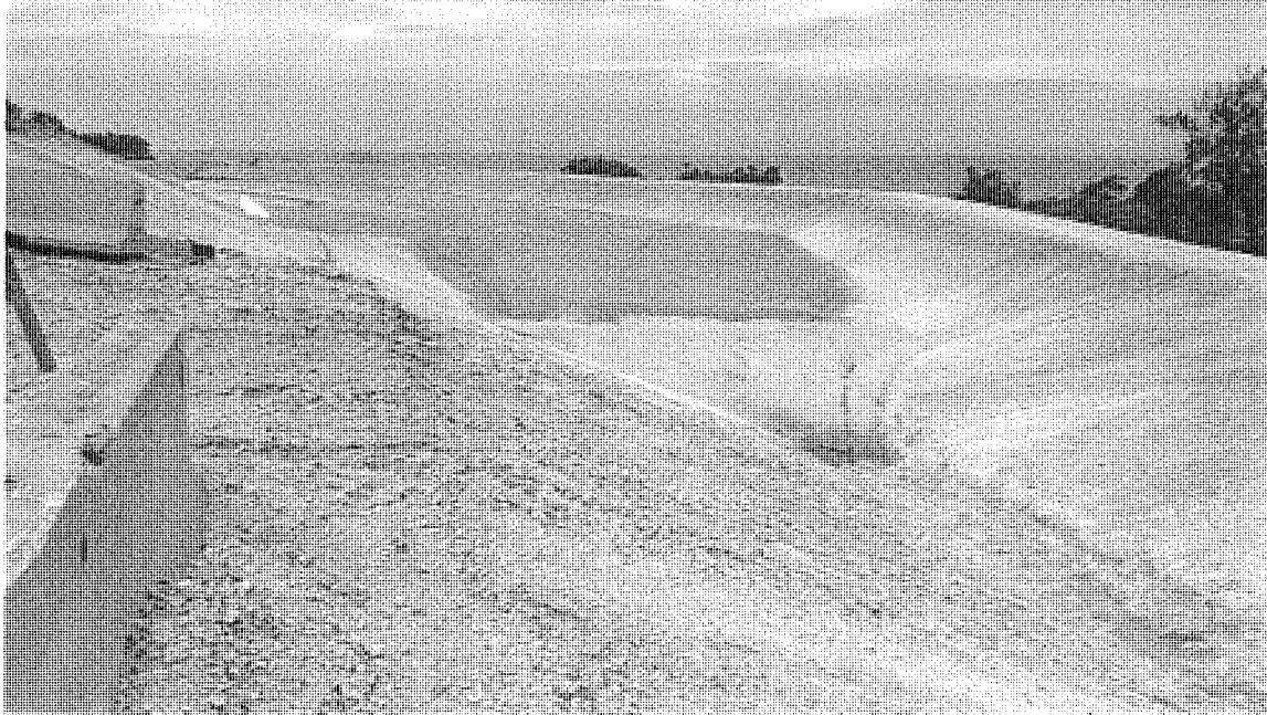
Pond 3. Overflow weir in distance is not yet finished – still requires stone riprap. (July 23, 2021)
